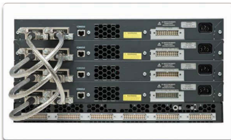
Stackable switches, connected by a special cable, effectively operate as one large switch.
