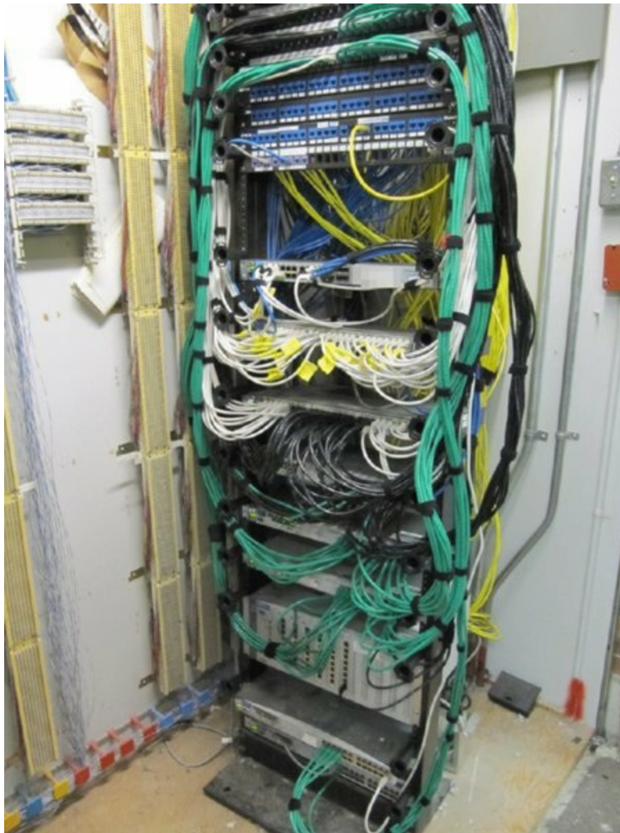
Figure 10.1 A typical wiring closet
