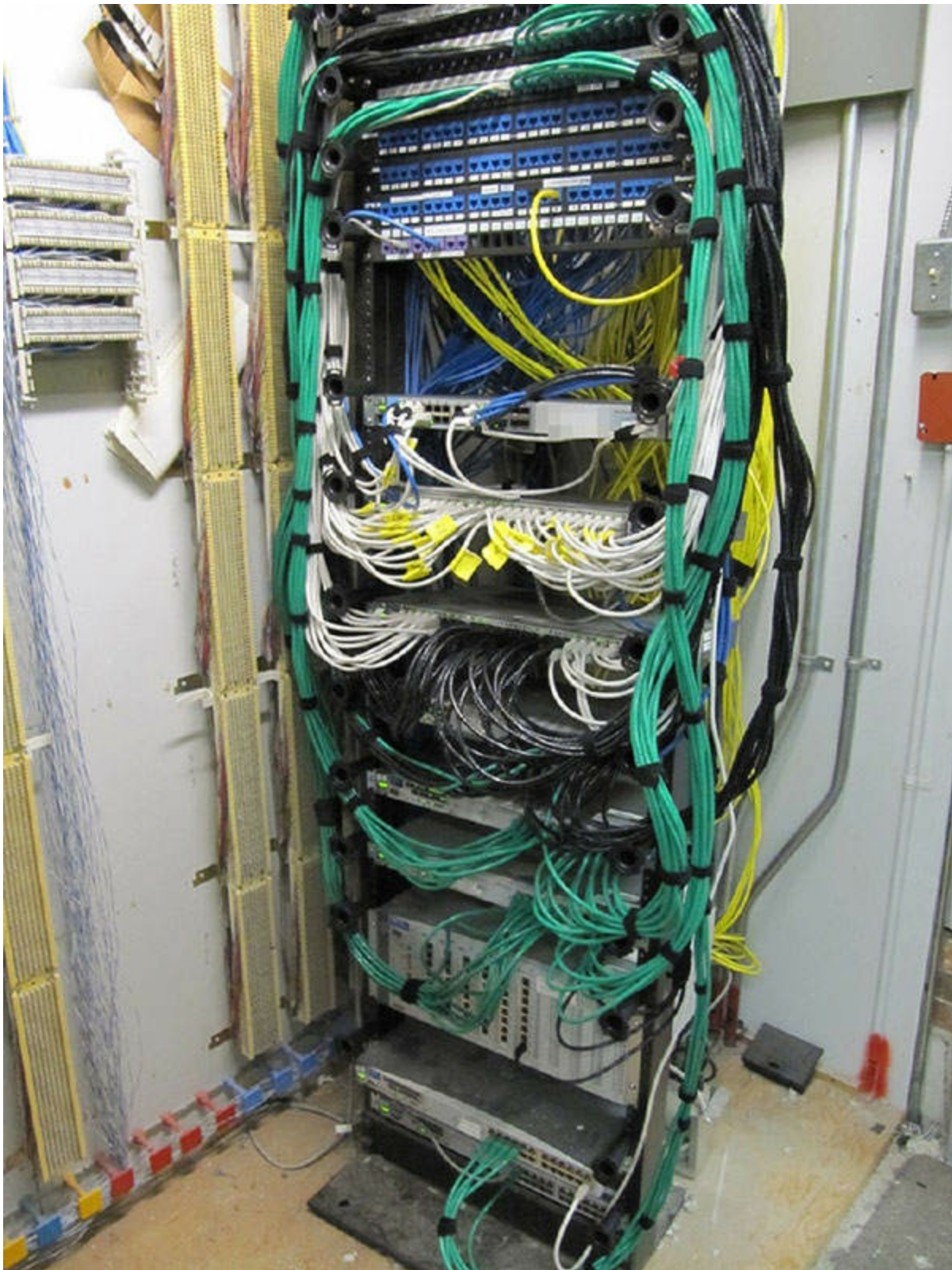
FIGURE 10.1 A typical wiring closet
